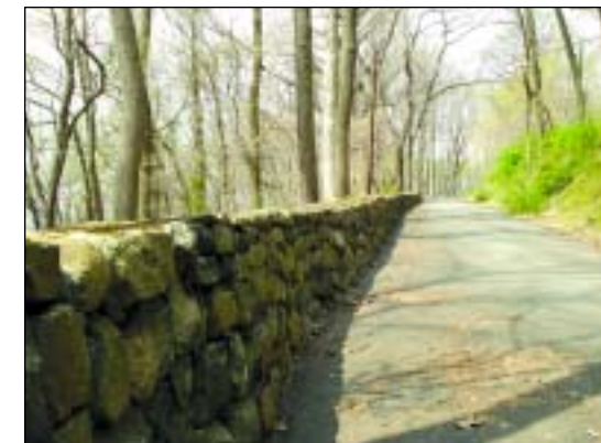
Paved roadway from Fiddlers Creek Road, leading up to the top of Baldpate Mountain.
