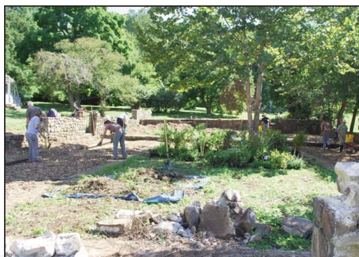
Staff and volunteers prepared the plots and planted native plants in September. The wall was still undergoing repair.
